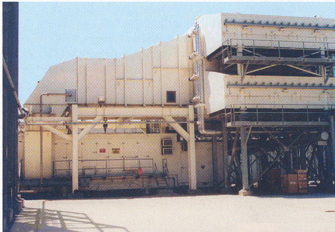
FIG. 1 A gas-fired GE 7EA combined cycle plant could raise gross profits by 43% by adding liquid fuel burning capability.
